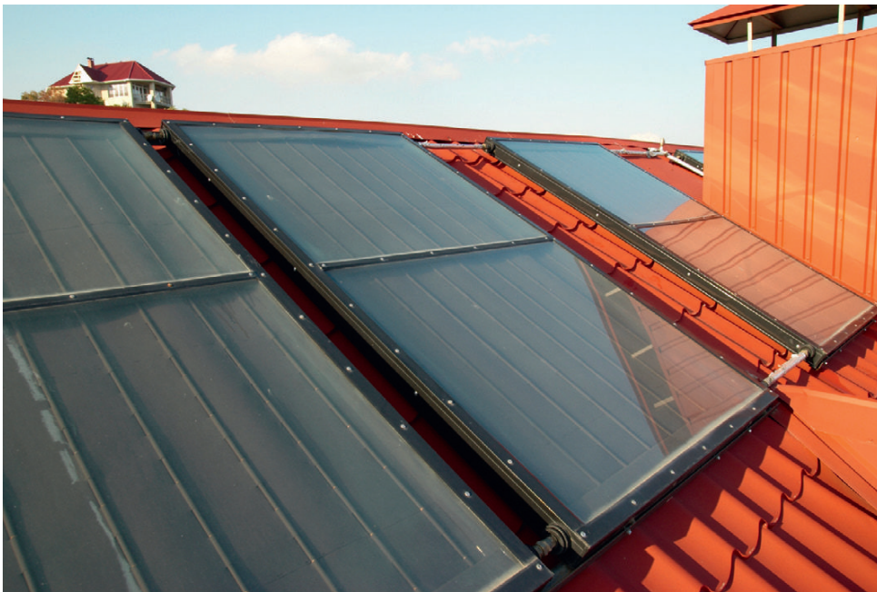
Figure 5.3 Photograph of a solar hot water panels.
