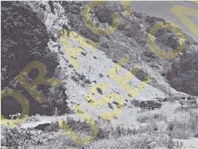
Figure 14.4 Repeated rock falls from the outcrop on this steep slope have created a fan of debris called talus . The road at the bottom of this slope must be cleared of debris following heavy rains, earthquakes, or other events. This slope is near Forest Falls, California (a place named for waterfalls, not rockfalls!).
