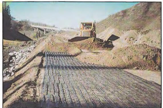
▲ Plate P Geogrid reinforced fill for a highway ( Tensar Earth Technologies, Inc. )
