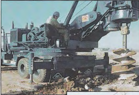
◀ Plate M Drilled shaft foundation under construction ( Association of Drilled Shaft Contractors )
