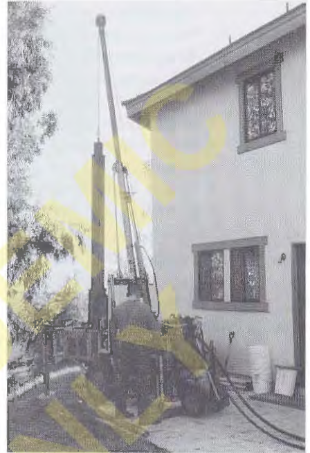
Figure 3.4 Limited access drill rig that can be moved through narrow openings. It is connected to a truck-mounted hydraulic pump via the hoses in the foreground.
