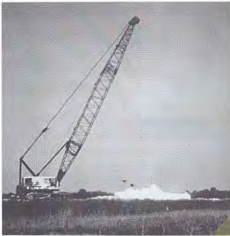
Figure 19.6 This crane is densifying the soil using dynamic compaction. It has just dropped a large weight onto the ground (GKN Hayward Baker, Inc.).
