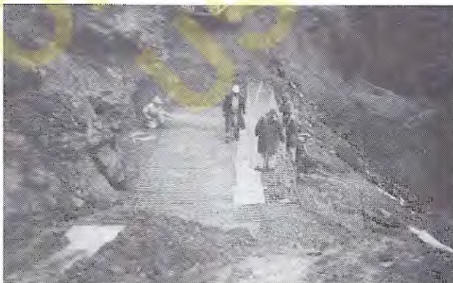
Figure 16.28 An MSE wall under construction using galvanized wire mesh as the tensile reinforcement and rock-filled cages called gabions for the facing (Federal Highway Administration).
