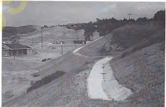
Figure 14.38 Typical surface drainage facilities on a cut slope. This concrete terrace drain captures surface water and carries it to a safe discharge point.
