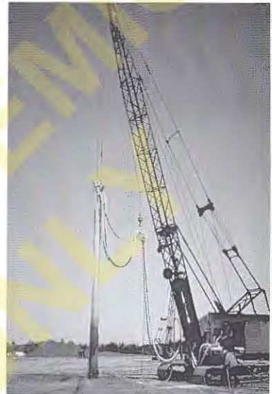
Figure 19.5 This crane is lowering a vibroflot into the ground (GKN Hayward Baker, Inc.).
