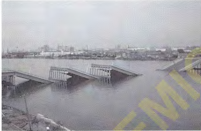
Figure 20.17 The Showa Bridge in Niigata, Japan, collapsed due to the formation of lateral spreads in the underlying soils during the 1964 earthquake. The lateral spreads moved the piers out of position, thus removing support from the simply supported deck. (Earthquake Engineering Research Center Library, University of California, Berkeley, Steinbrugge Collection)
