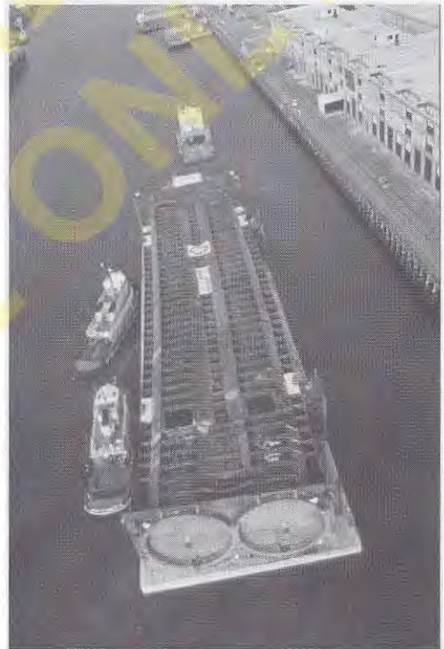
Figure 11.28 This prefabricated tunnel section is part of the Central Artery Project in Boston. It was floated into position, then sunk to the bottom of the bay (Photograph by Peter Vanderwarker, courtesy of the Central Artery/Tunnel Project).
