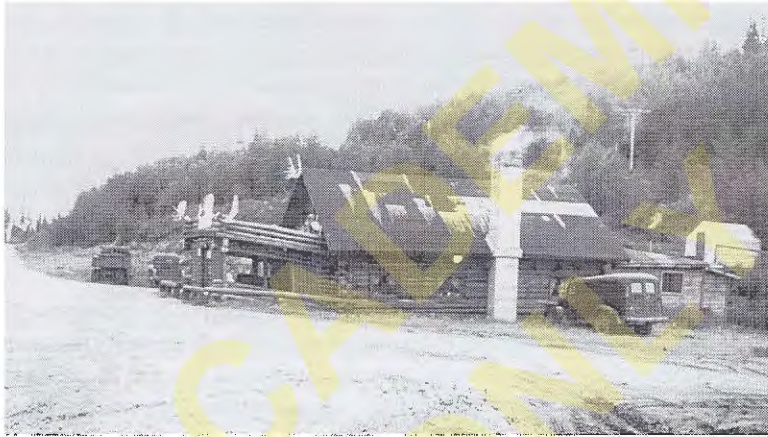
Figure 18.6 Heat from this lodge in Alaska thawed the permafrost below, causing it to settle. However, the permafrost did not thaw beneath the unheated porch (Photo courtesy of Professor Richard L. Handy).
