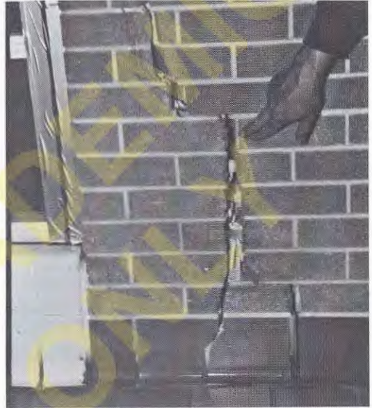
Figure 18.1 Heaving of an expansive soil caused this brick wall to crack. The $490,000 spent to repair this and other walls, ceilings, doors, and windows represented nearly one-third of the original cost of the six-year-old building (Colorado Geological Survey).
