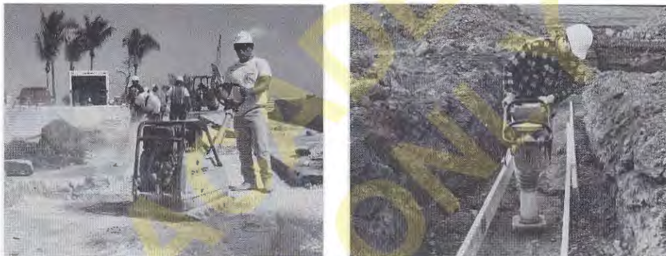
Figure 6.25 Using portable compaction equipment to compact soils in areas that are too confined to accommodate large equipment (Wacker Corporation).
