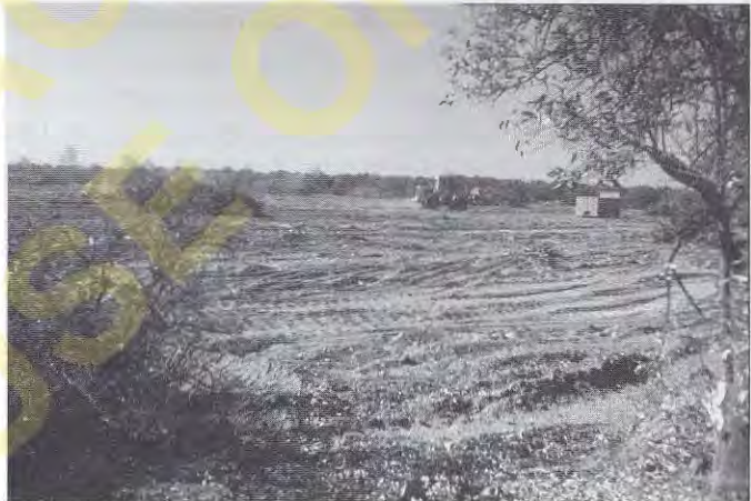
Figure 6.10 Clearing and grubbing in a former orange grove. The trees are being removed and hauled to the dumpster seen in the background.
