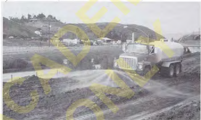
Figure 6.18 A water truck spraying a new lift of soil for a fill and preparing it to be compacted.
