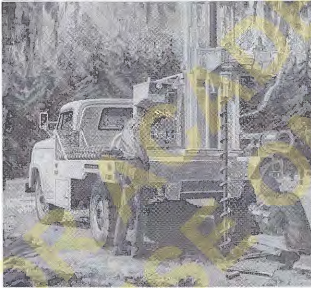
Figure 3.6 A crew drilling an exploratory boring using a truck-mounted flight auger. These augers typically have an outside diameter of 120–200 mm (3–8 in). (Foremost Mobile Drilling Co.)
