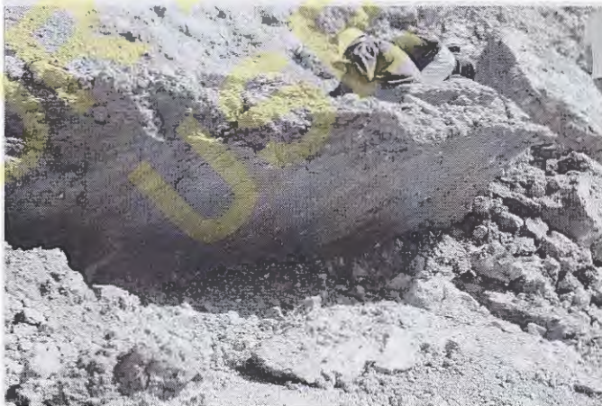
Figure 13.22 This slickenside was formed by a landslide in a clay. The shear strength along this surface has been reduced to the residual value.
