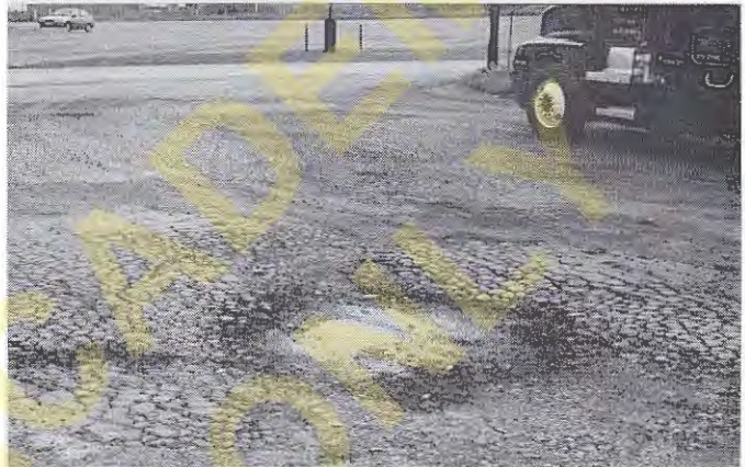
Figure 18.4 The soils beneath this asphaltic concrete pavement in New York became wet and soft during the spring thaws. As a result, these soils failed under the weight of the heavy trucks that use this site. The pavement is now in very poor condition, with extensive alligator cracks and potholes.
