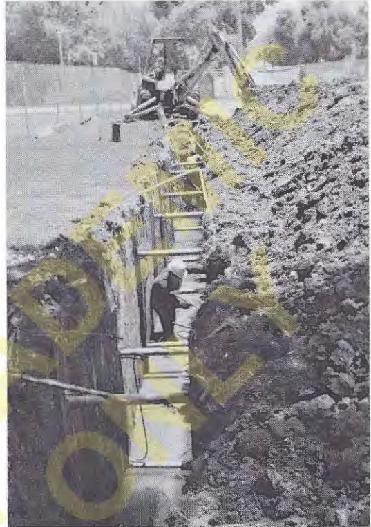
Figure 3.15 This exploratory trench was dug by the backhoe in the background, and has been stabilized using aluminum-hydraulic shoring. An engineering geologist is logging the soil conditions in one wall of the trench. In this case, the purpose of the trench is to locate a fault.
