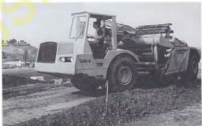
Figure 6.11 A scraper transporting a load of soil across a construction site. This scraper is equipped with an elevating mechanism at the front of the bowl to assist in loading soil.
