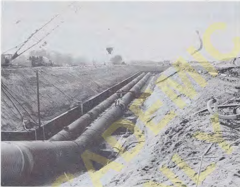
Figure 8.28 This 11 m (35 ft) deep excavation was required to construct these two water supply pipelines. The excavation extends 10 m (35 ft) below the groundwater table, and a river is located just beyond the excavation on the left side of the photograph. Therefore, a temporary dewatering system has been installed to draw down the groundwater table. This system includes a series of pumped wells, including the one in the right foreground (Photo courtesy of Foothill Engineering).
